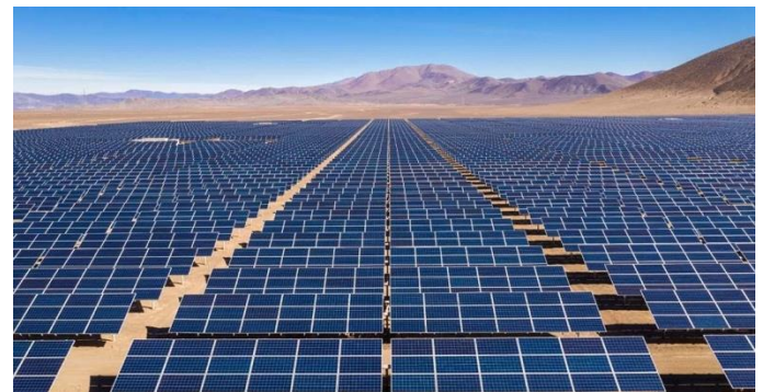
Figure 9. SEFA Solar Panels https://www.eqmagpro.com/afdb-sefa-grants-760000-to-develop-small-scale-renewable-energy-projects-across-sub-saharan-africa/
